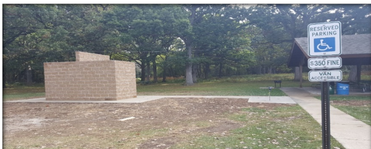
Accessible sidewalk to shelter and new restroom, with accessible water hydrant at Fabyan East. Project completed in-house by Trades Division.
