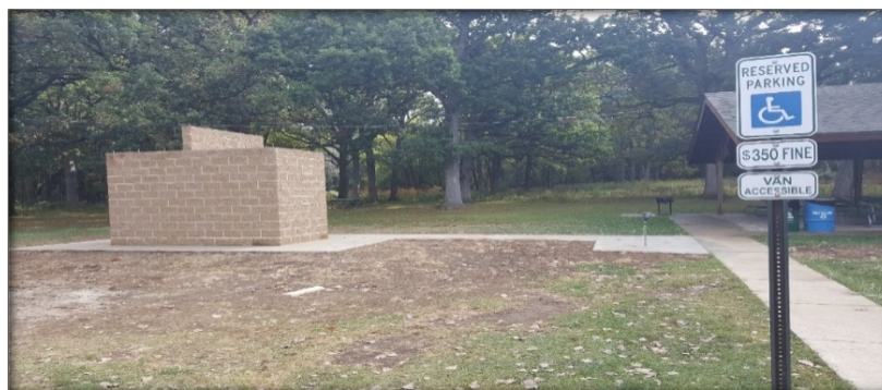
Accessible sidewalk to shelter and new restroom, with accessible water hydrant at Fabyan East. Project completed in-house by Trades Division.
