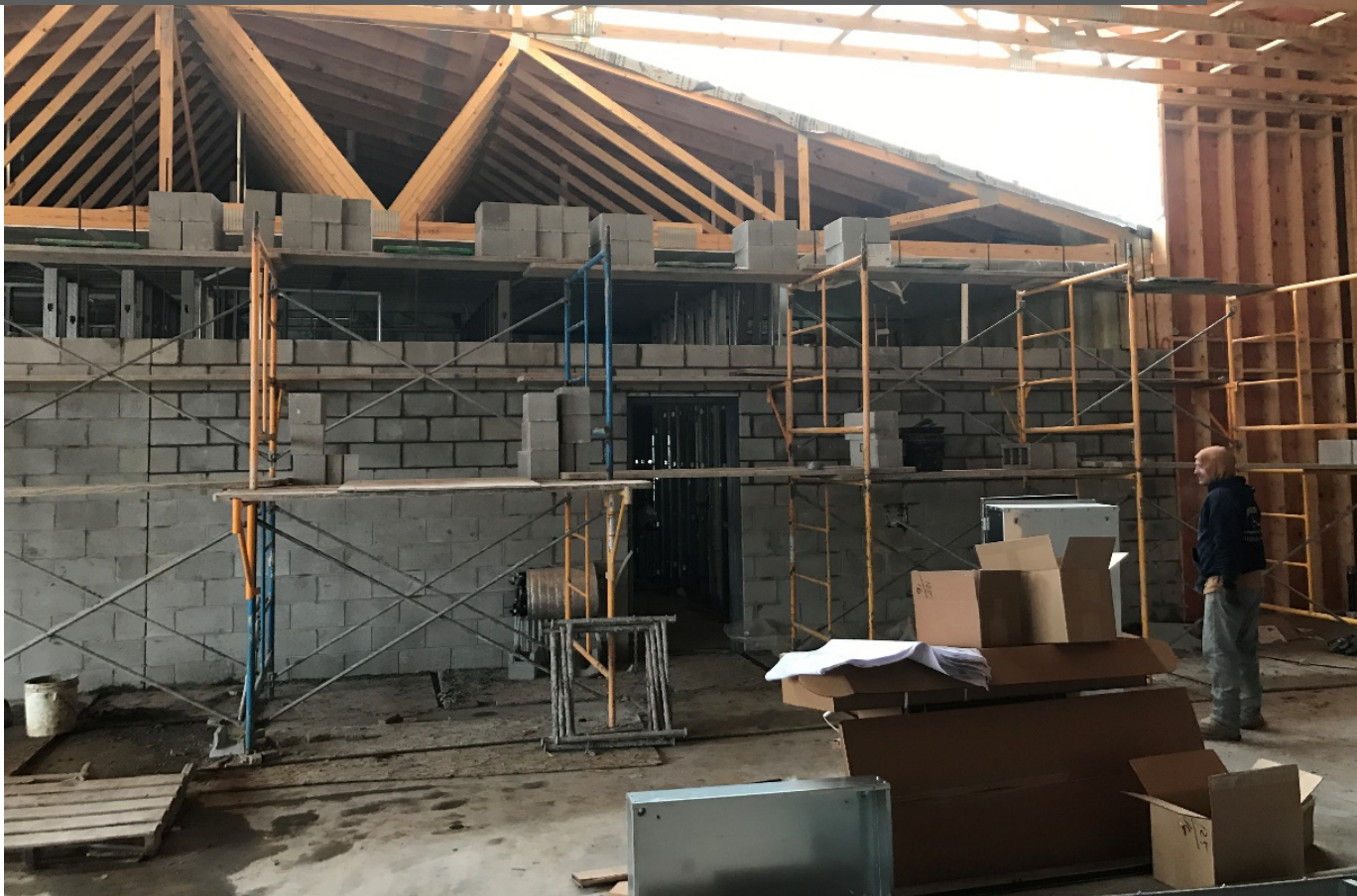
Photo of the Natural Resources Facility Under Construction at Mill Creek Greenway, Credit to Benjamin Haberthur.
